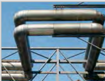
Pipelines subject to pressure
